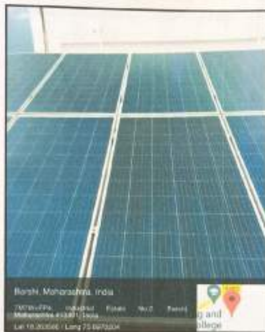
Photograph of Roof Top Solar PV Plant:
