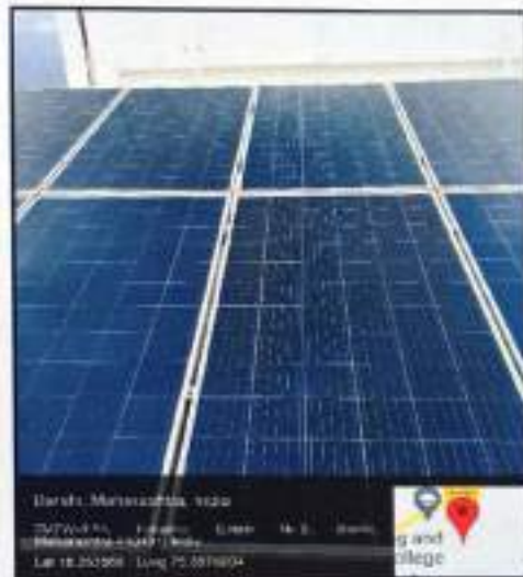
Photograph of Roof Top Solar PV Plant:
